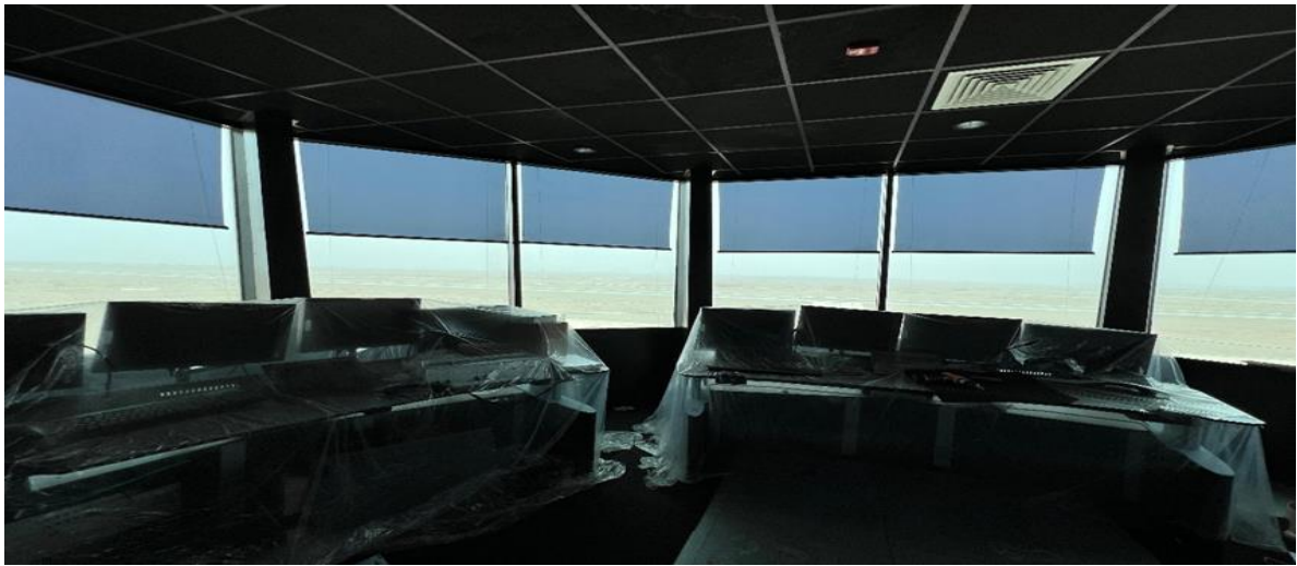
Figure - 9 showing the equipment fitted in the unmanned Control Tower viewing east direction
